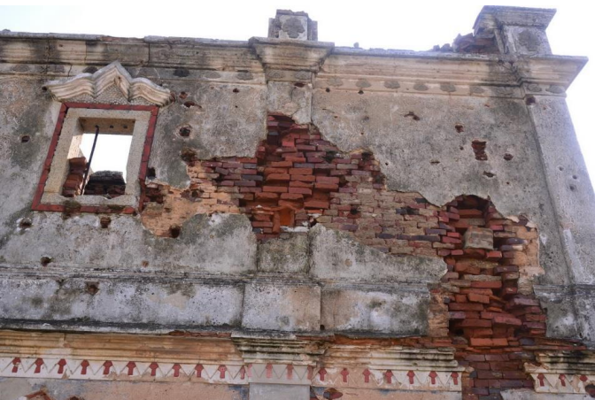
Deterioration of plaster walls
