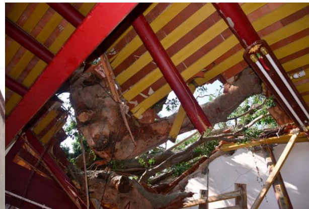
Fallen banyan crashed the roof
