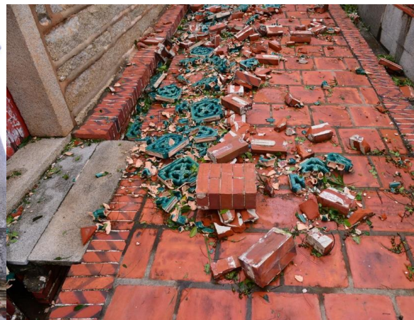
Fragments of a crumbled parapet
