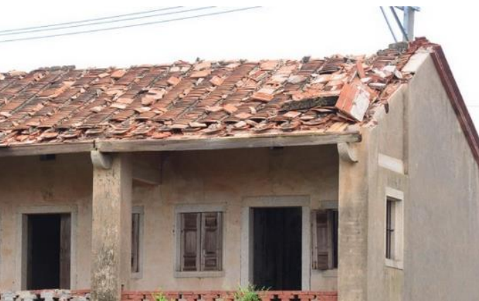
Loosened roof tiles caused by windstorm
