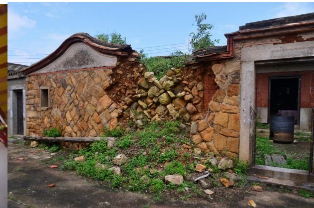
Disintegration of wall
