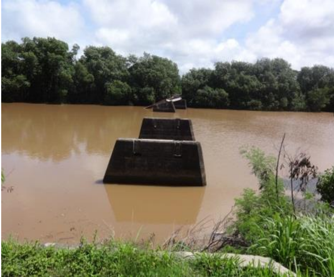
Hurricane Destroyed Railway Bridge Natadola Image: Chris Richards 2016
