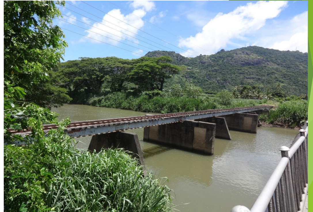
Rail Bridge number 29 over the Nadi River Source: Chris Richards 12th February 2016
