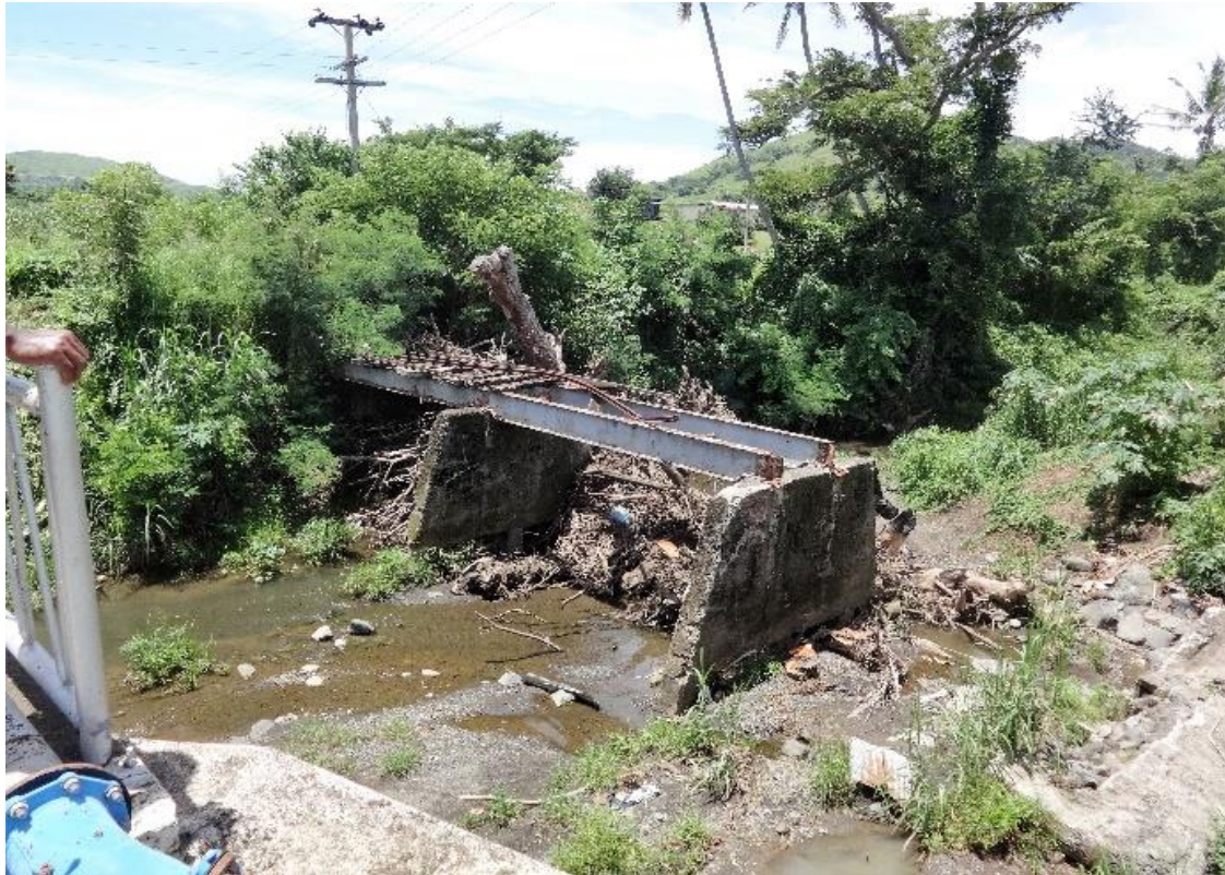
Hurricane Winston Damaged Railbridge Penang Sugar Mill Image: Chris Richards 2016
