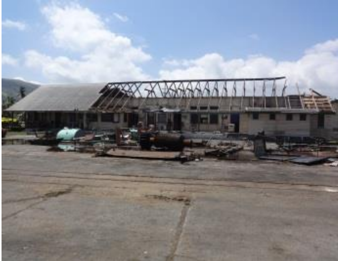
Hurricane Winston Damage Penang Sugar Mill Image: Chris Richards 2016
